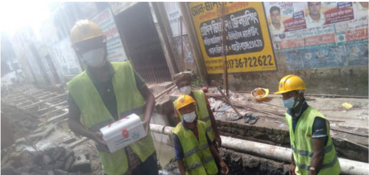
“First Aid Box” at a Road work site in Brahmanbaria Pourashava area
